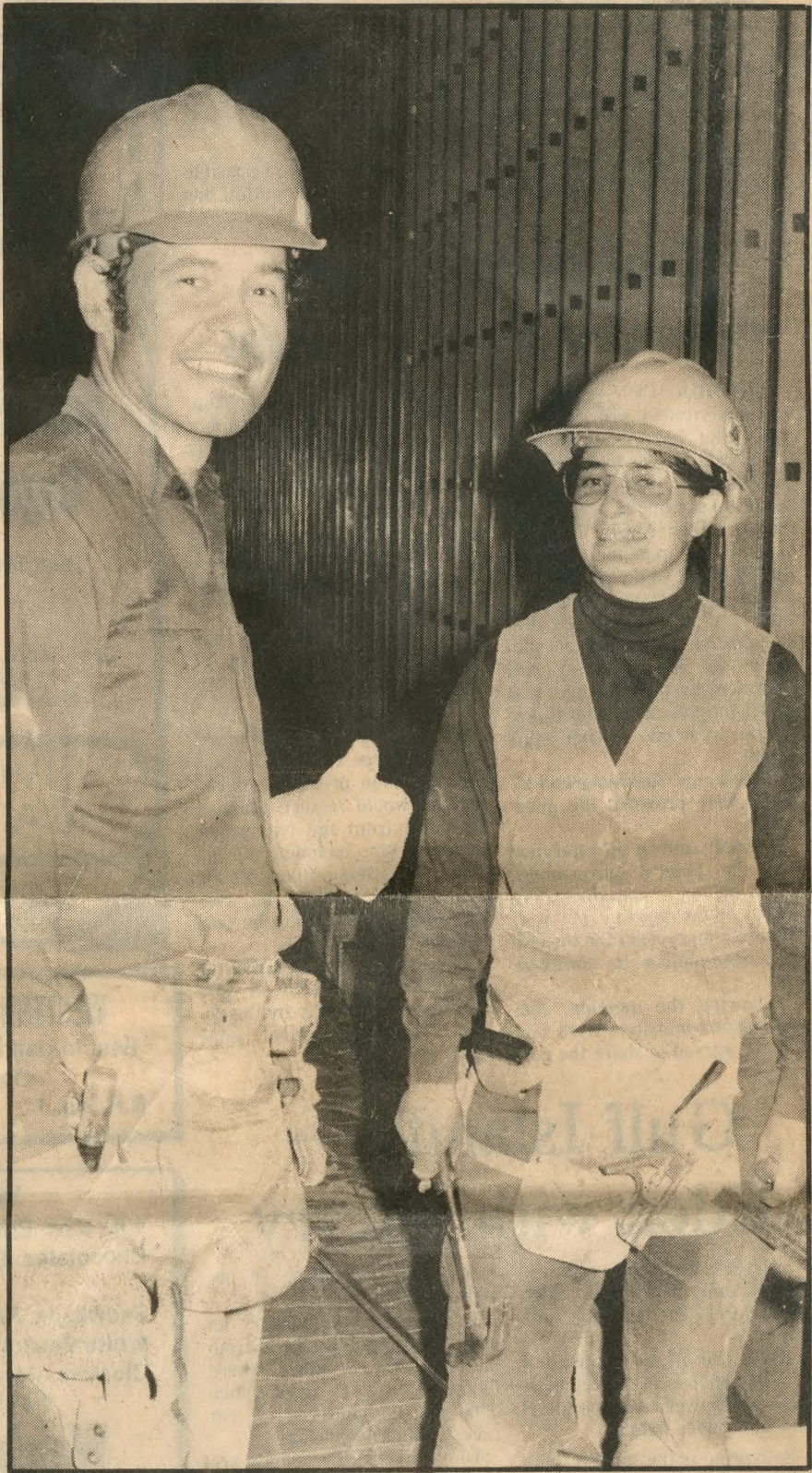
IF I WERE A CARPENTER — Alex Chernoff of Krestova takes a stretch while building cement forms with co-worker Marcia Braundy at Nelson's Chahko-Mika mall. Chernoff's union, Local 2458 of the United Brotherhood of Carpenters and Joiners of America, recently voted Braundy in as the first unionized woman carpenter in B.C.
